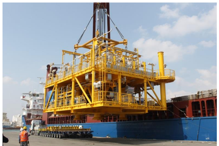
CSP (Conductor Supported Platform) topsides being loaded into the Industrial Force vessel for transportation to Cotonou
